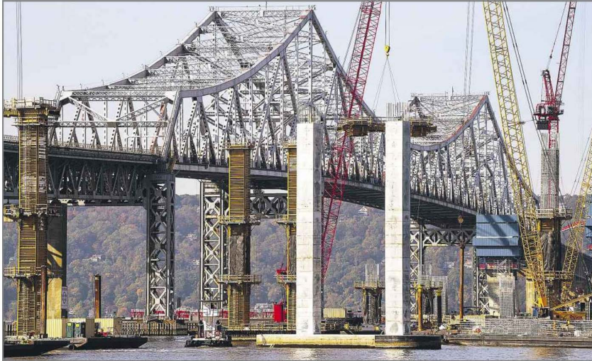
The old Governor Malcolm Wilson Tappan Zee Bridge, with parts of Governor Mario M. Cuomo Bridge.
