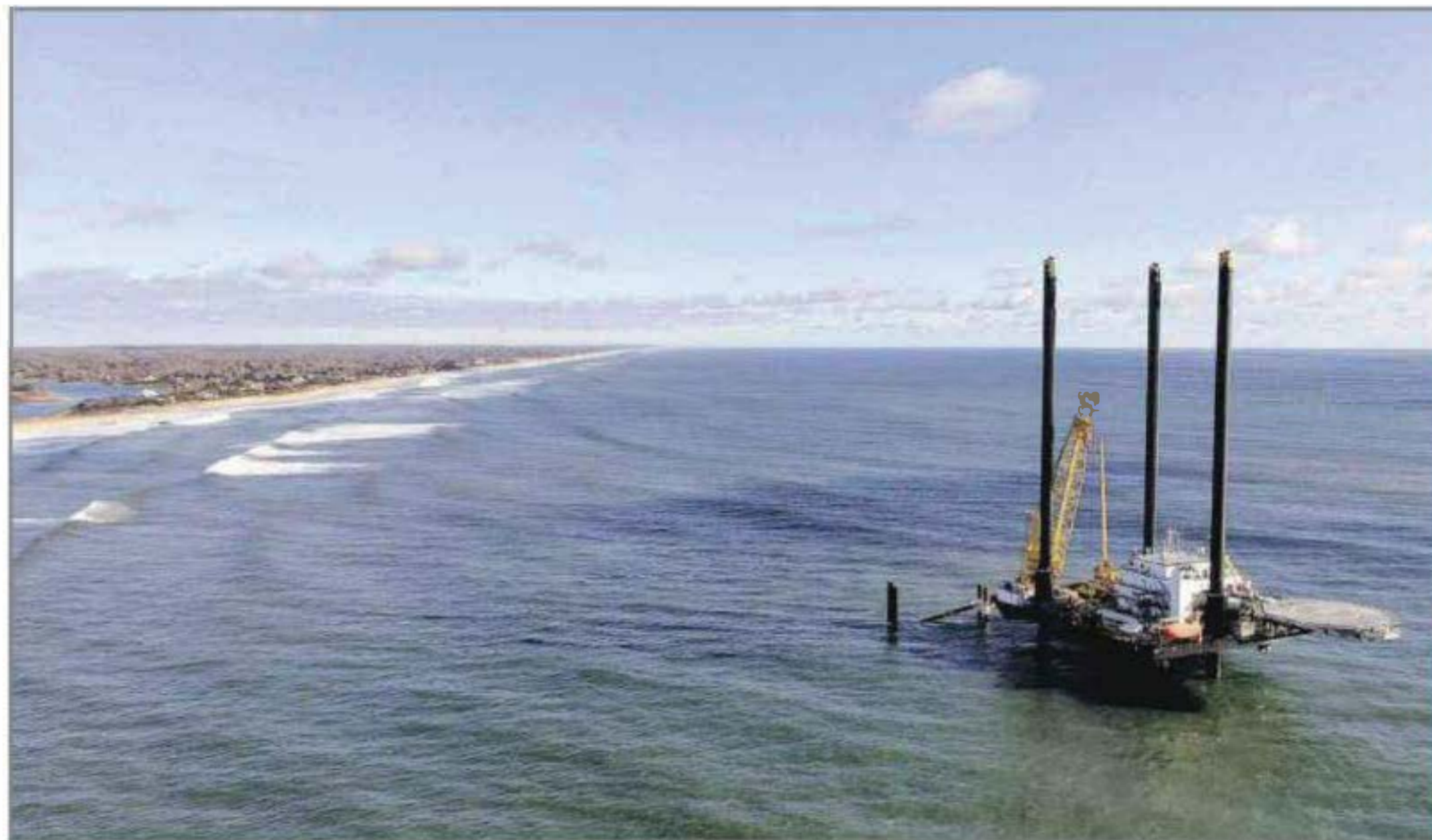
A vessel such as this is used to lay a wind farm's power cable connection to land infrastructure.
